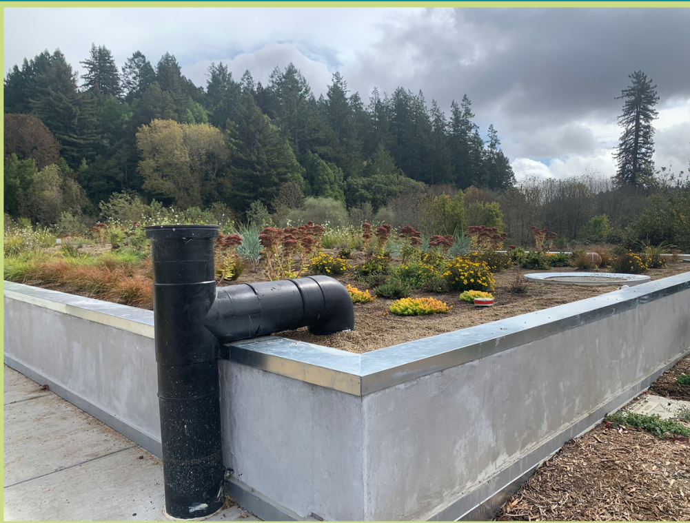
Salmon Creek water cistern and living roof
